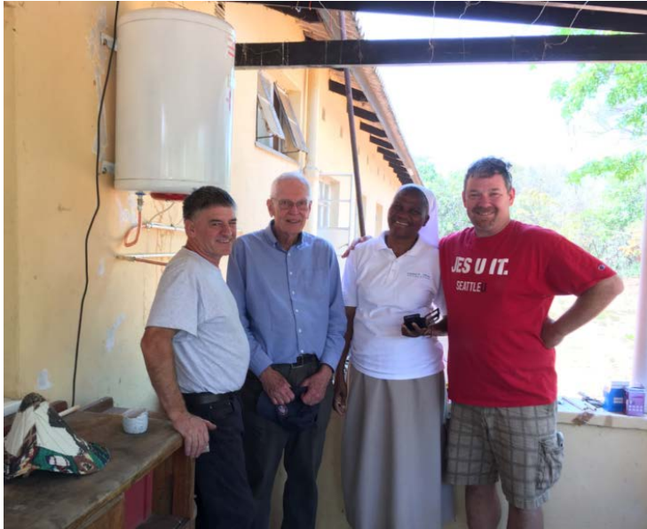
Providing and installing a new (Geezer) hot water tank for the Sisters of the Holy Spirit with the assistance of Fr Bert Otten S.J.
